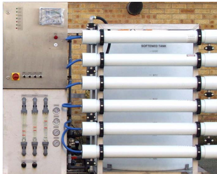
Figure 17: Filter Connected to a Control System
