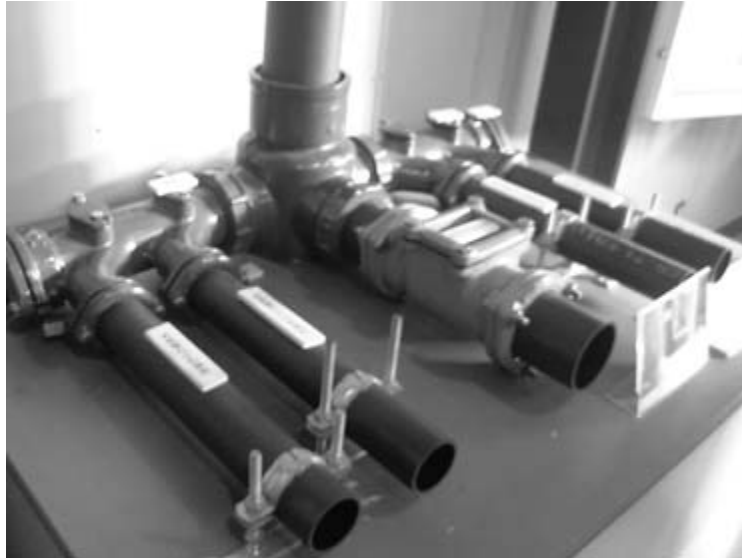
Figure 11: Sewage header of KSI
