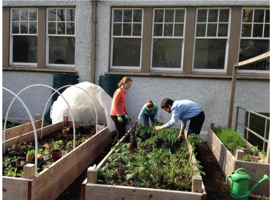
Figure 8: Installation of planter boxes in front of the Geography Building at the UBC Point Grey Campus, 2013.
