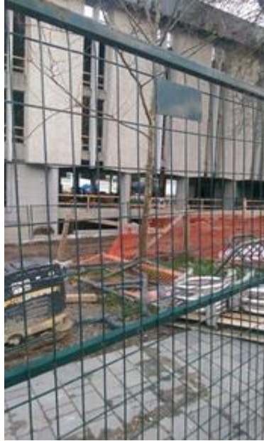
Figure 1: Broken tree protection fencing on University Boulevard
