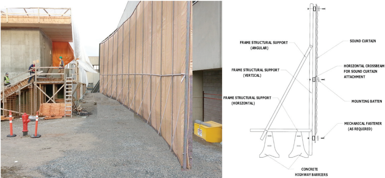
Figure 5. Left: rendering of a noise barrier setup for the CEME classroom. Right: section of the noise barrier. Source: All Noise Control, n.d.
