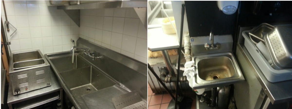
Figure 1: Main Floor Kitchen Double Sink (left) and Hand Sink (right)
