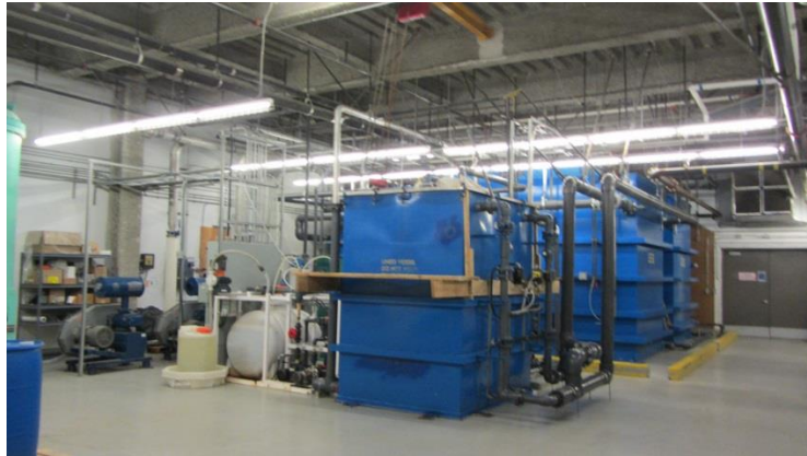
Figure 3: Water treatment Facility of Vancouver Convention Centre
