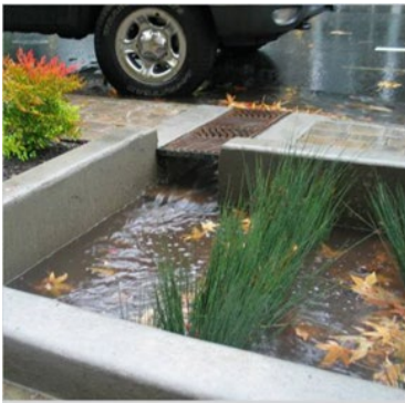
Figure#19 Street runoff enters planter (Photo by Kevin Perry, Bureau of Environmental Services, City of Portland)
