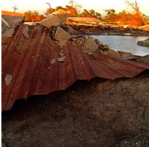
Figure 13: Rotational failure of wall (Levees.org).
