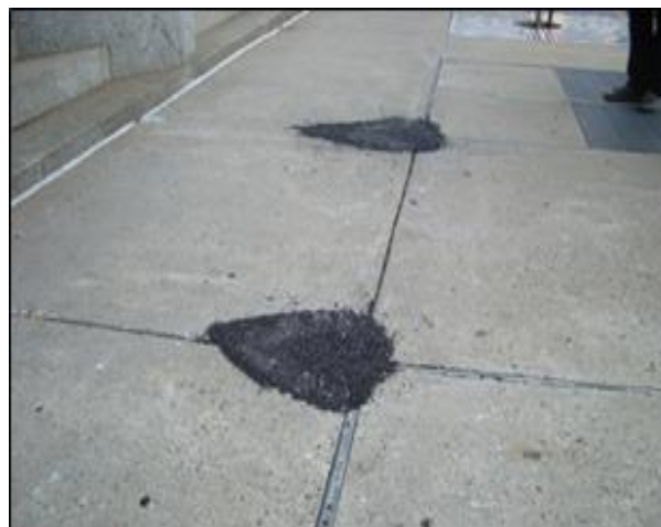
Figure 9: An asphalt patch applied to help smooth out the uneven pavements
