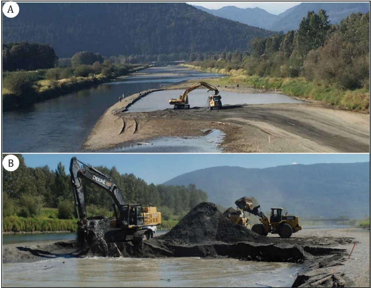
Figure 5 Excavation of gravel bars in in Vedder River and Canal (A) leaving irregular bar surface and local increased turbidity (B). [Photo by VERMAC (A), Jakes Construction Ltd. (B)]
